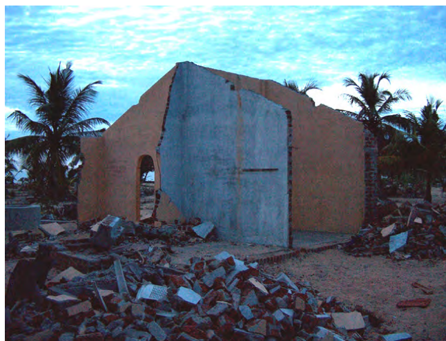
The devastation zone - 6 months after the Tsunami. Kalkady, Batticaloa
